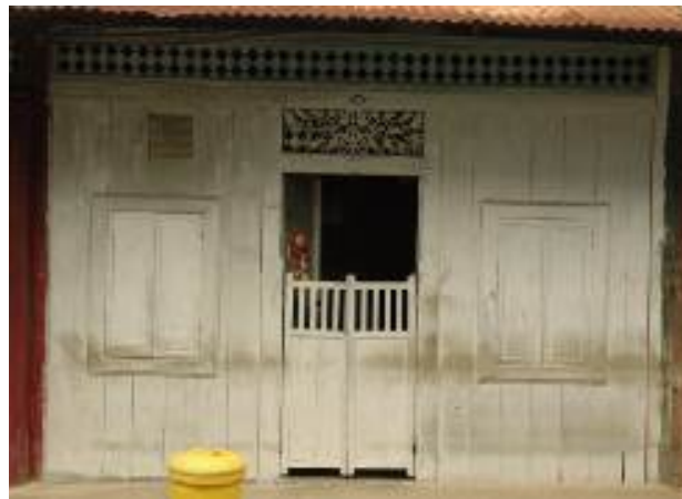
Figure 1 A wooden Chinese shophouse still existing in Kota Bahru, Kelantan. The ground floor entrance is affixed with a plain half-door or pintu pagar before another full door, which is opened from the inside, the pintu pagar being a typical Malay architectural feature. On top of the door is an intricate wood carved rectangular-shaped vent of Malay influence (Photograph by the author).
